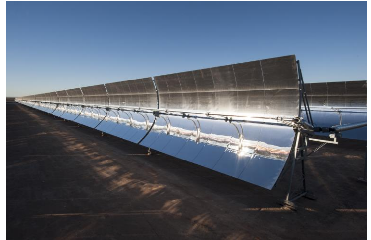
Solana Solar W/Thermal Storage
